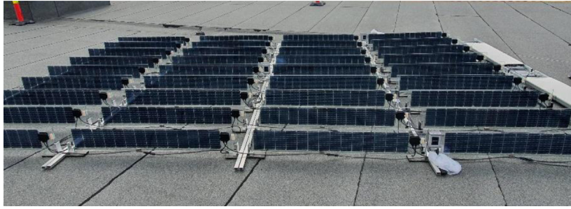
Fig. 1. The Over Easy pilot installation at Institute for Energy Technology, Kjeller, Norway.
