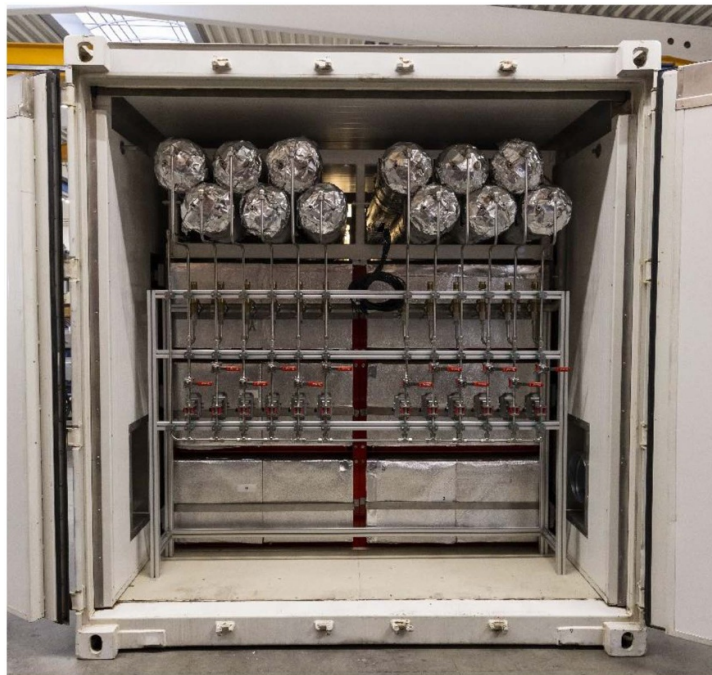
Figure 23. HyCARE system: cylinders at the top contain the metal hydride for hydrogen storage and boxes at the bottom contain the PCM for heat storage.
