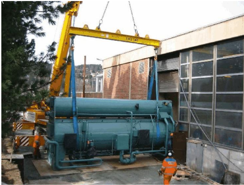
- Figure 4: The absorption chiller at Øya Cooling Central. Source: Trondheim Energi
