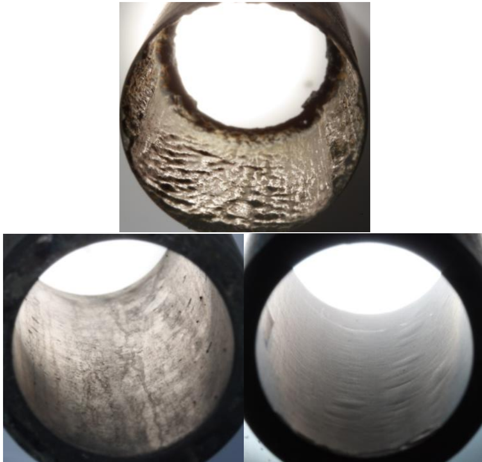
Figure 1 Comparison of carbon steel surfaces exposed to unmitigated CO 2 corrosion (upper image) and protected by inhibition (lower left) and pH stabilization (lower right)
